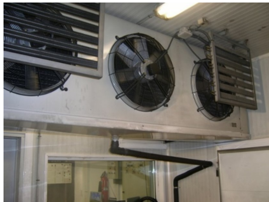
Figure 6.2: Photograph of room conditioning system.
