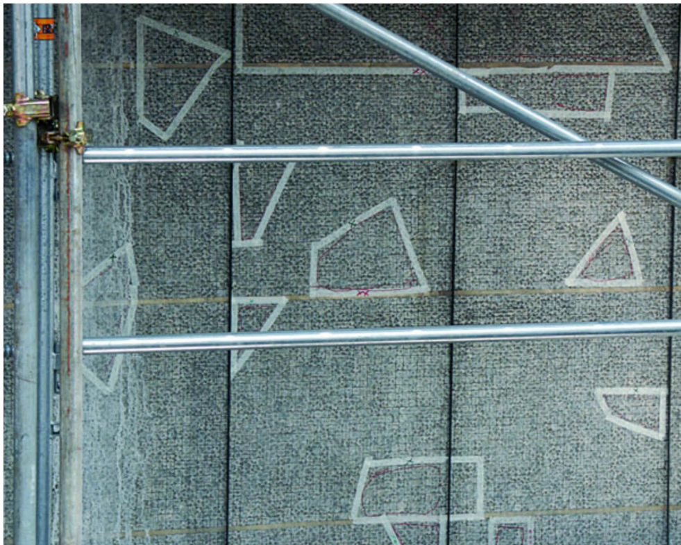
Figure 5.12: Mapping of missing ceramic tiles. Source: Il restauro del grattacielo Pirelli a Milano [32].
