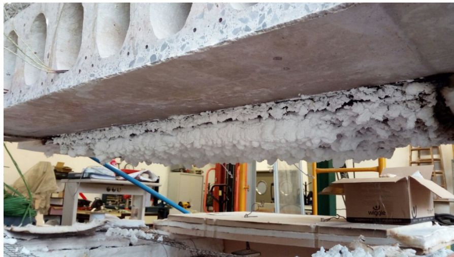
Fig. 9. View of A6 specimen from its bottom surface after fire exposure.
