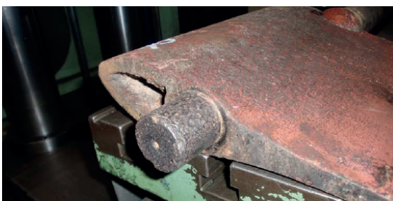
Figure 9: Detail of damage to turbine distributor blades due to cavitations. (Source Endesa Generación-Enel Green Power).
