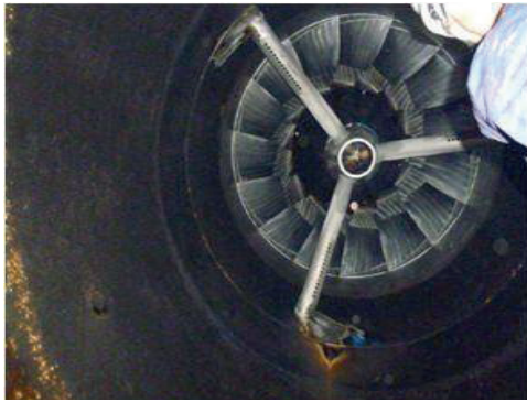
Figure 12: Detail of turbine cone aeration pipes due to cavitations. (Source Endesa Generación-Enel Green Power).
