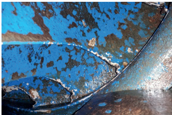
Figure 8: Detail of turbine damage due to cavitations. (Source Endesa Generación-Enel Green Power).
