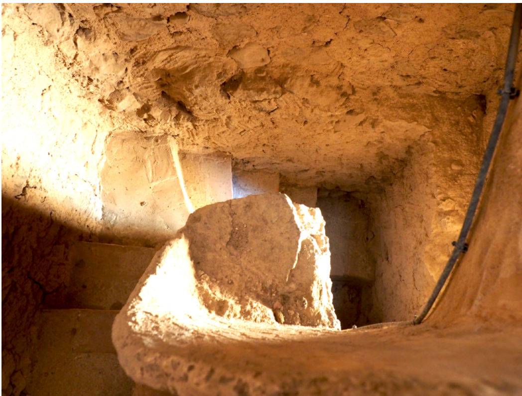
Figure 18. Lateral wall of the 13 th century bell tower, the bottom of which used the buttress of the diaphragm arch to close the structure (exploration 1). Source: authors
