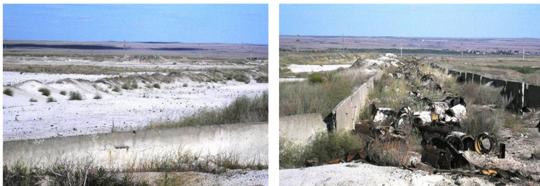
Figure 4 – Pipeline condition with traces of emergency discharges
