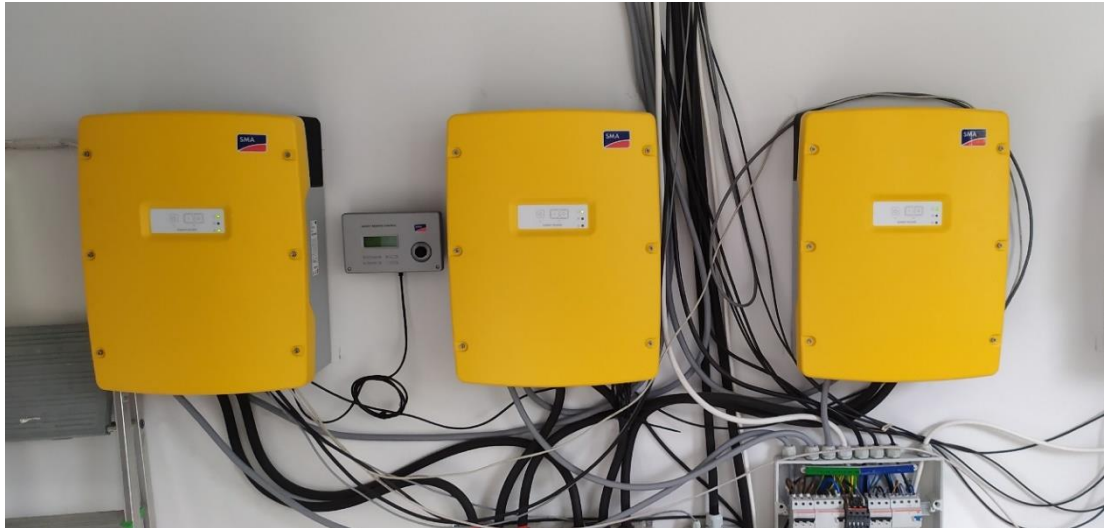
Figure 14: Three Sunny Island bidirectionals inverters. Master inverter on the right and two slaves inverters on the left and the Sunny Remote Control between the master and the first slave inverter
