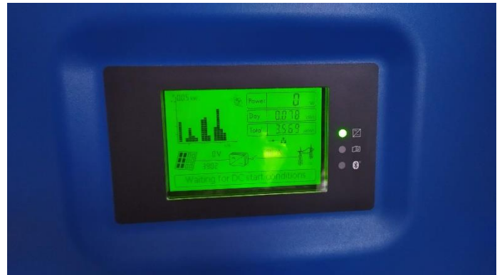
Figure 7: Display detail of Sunny Tripower inverter
