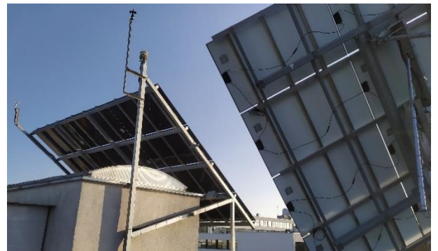
Figure 5: Structure of both solar power plants
