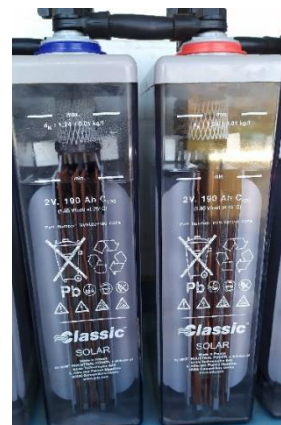
Figure 13: Detail of a battery of 2 V
