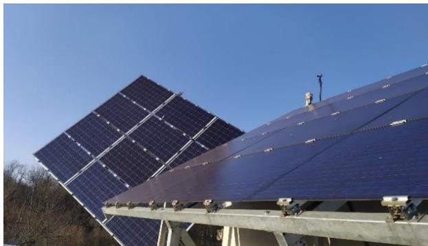
Figure 4: Front of the two solar power plants
