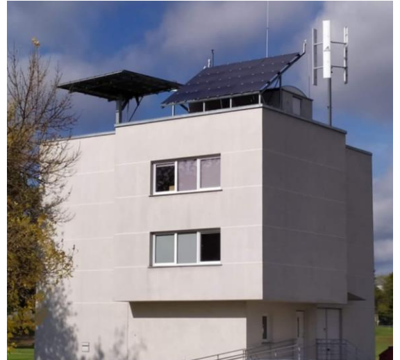
Figure 2: Laboratory building with the different generators of the microgrid on the roof
