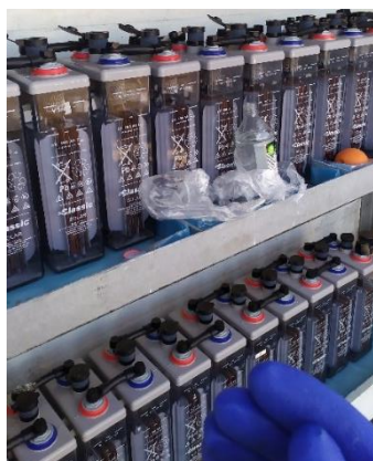
Figure 12: Battery set of the microgrid
