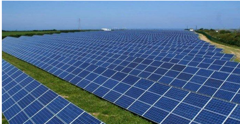
Figure 17. PV generator integrated by the interconnection of pv modules. Source: Portal Energía
