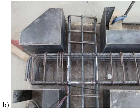
Figure 7. Instrumentation. a) Strain gage layout in joints, b) strain gages in Joint 2 steel cage.
