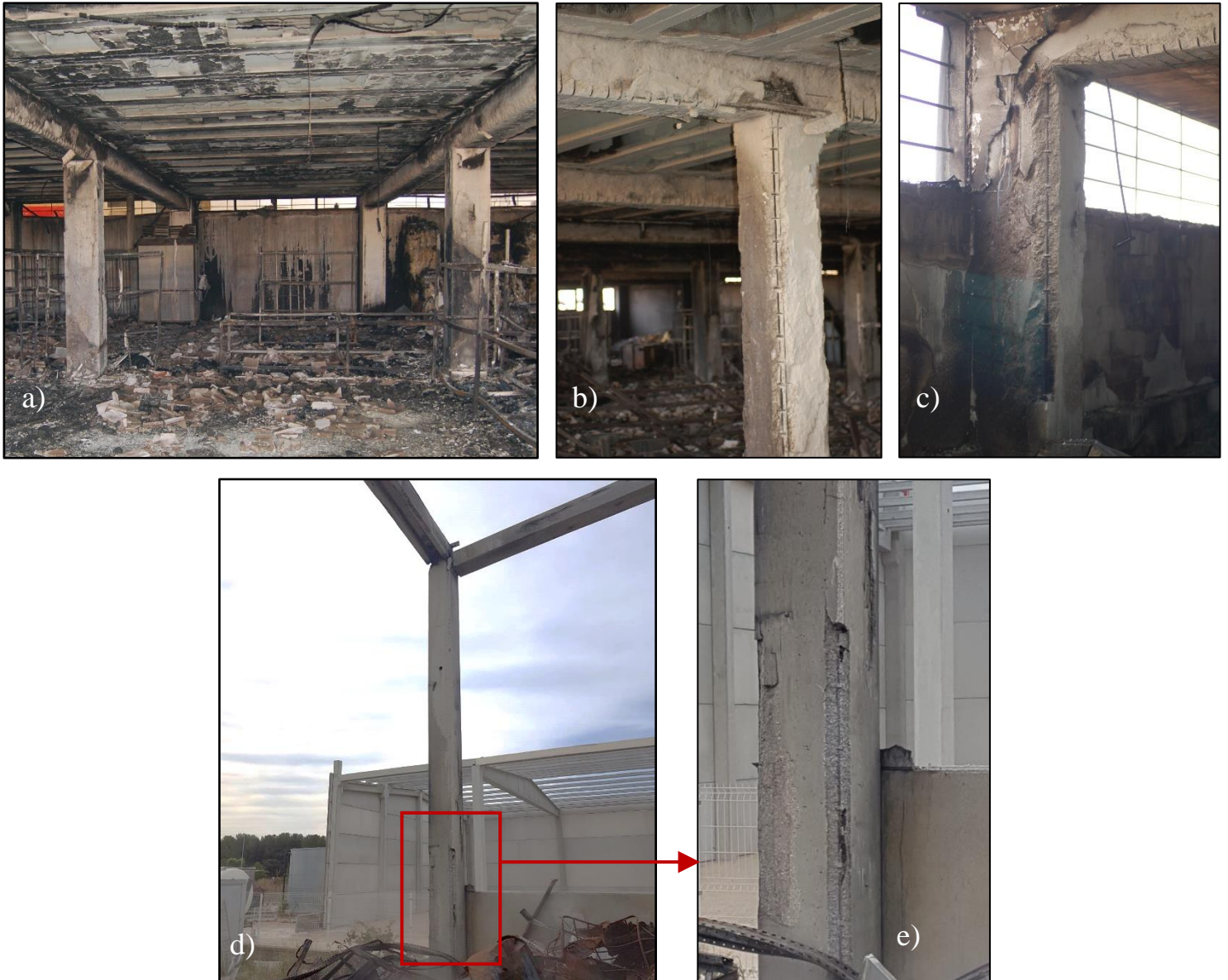
Fig. 1. a) RC industrial building after a fire; b) Column after a fire (corner spalling); c) Lateral column after a fire; d) RC corner column at industrial building after a fire; e) Detail of spalling in RC corner column.
