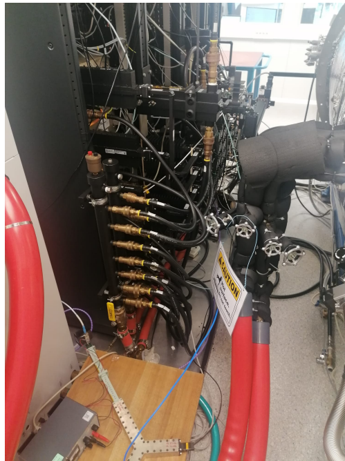
(b) Rear view - Multiplexer and PIM filters.
