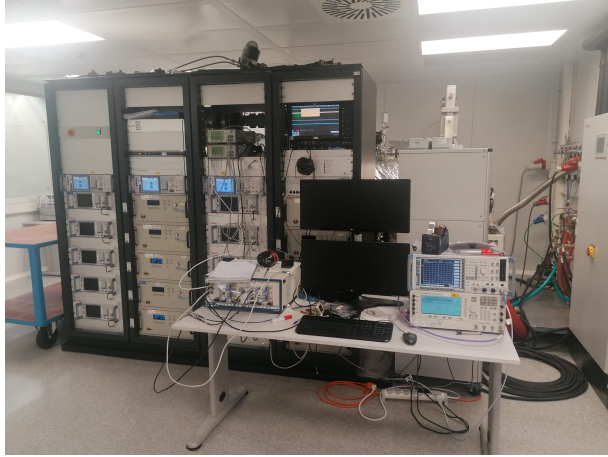
(a) Front View - Signal generators and HPAs.
