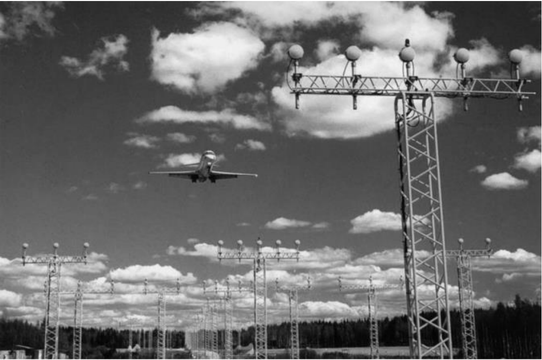
Figure 16 Typical airport approach lighting assemblies (Courtesy, Exel Oy, Finland)
