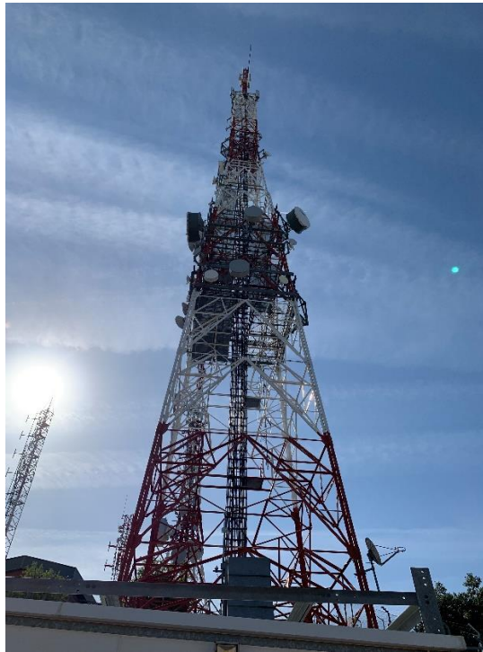
Fig. 29 High Power High Tower used in TelecomCLM pilot
