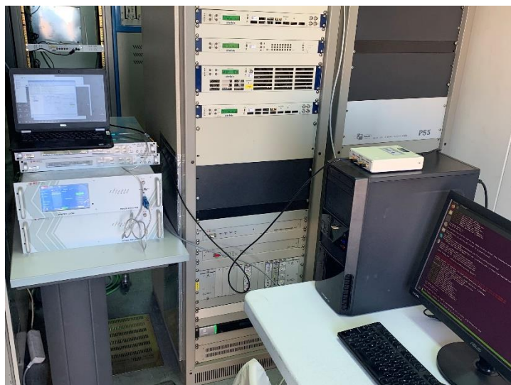
Fig. 28 TelecomCLM pilot deployment in Toledo
