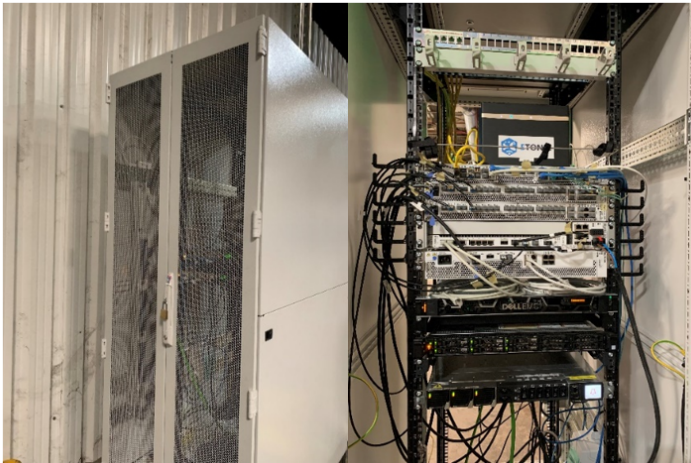
Figure 110: 5G Rack inside a protection cupboard at Ford factory.
