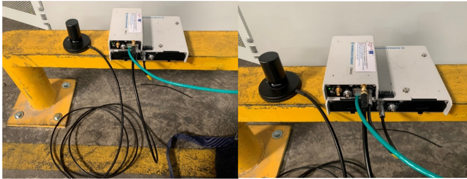
Figure 113: Coverage measurement equipment.
