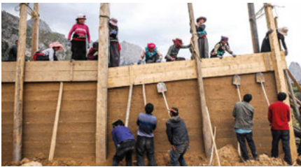
Fig.6 People were pushing up side planks of the integral formwork (Source: Shu, 2016, https://www.poco.cn/works/detail_id5245000 )
