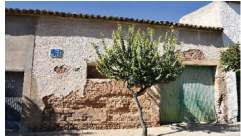
Fig. 6. Vernacular adobe building with visible erosion.
