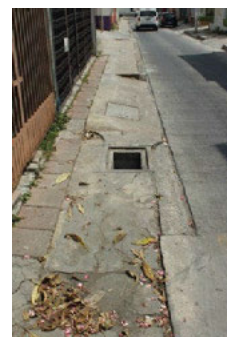
Fig. 2. Sidewalk of the neighborhood in deplorable condition. (Source: Parra Zebadúa, 2021)
