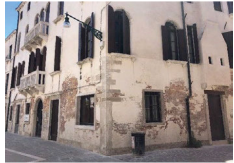
Fig. 5. New thick plasters cannot withstand the effect of rising damp for long in Venice: the above example is less than a decade old (Source: Squassina, 2021)
