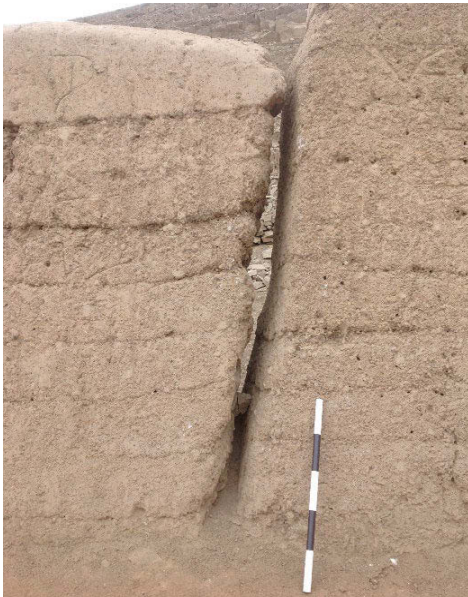
Fig. 2. Mud layers in a wall, it can see the concavity formed. Palace of Oquendo – Lima (Source: Torres, 2021).
