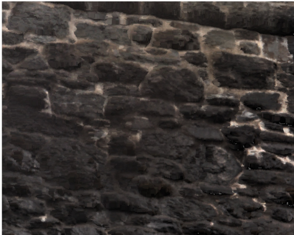
Figure 6. Typical section of the RGB textured point cloud. Only slight differences between joint and stones are visible, mineral efflorescence disturbs the joint pattern.
