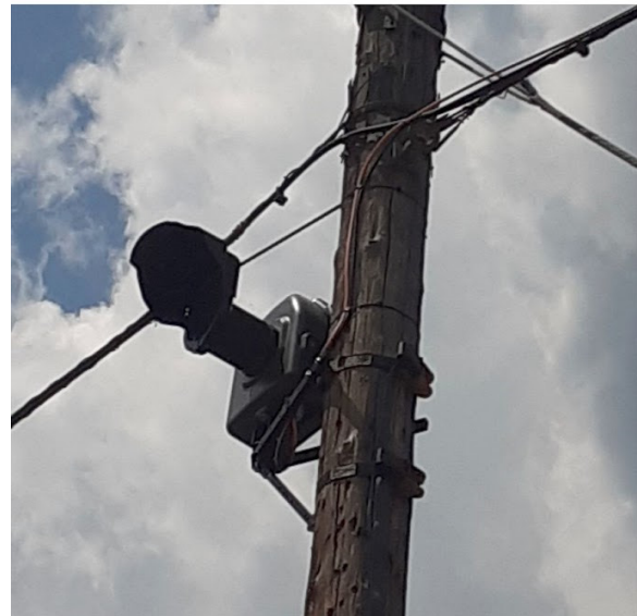
Figure 3. Top: Control unit next to Camera 2 (C2). Bottom: Camera 3 (C3) placed on a telecommunication wooden pole.
