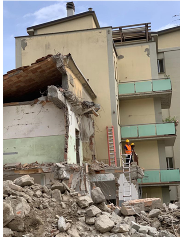
Figure 1. The wall to be monitored adjacent to the building to be demolished.
