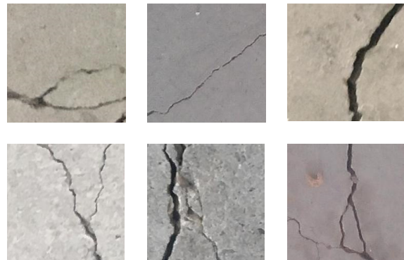
Figure 2. Examples of cracked surfaces ("Positive") (Özgenel, 2019).
