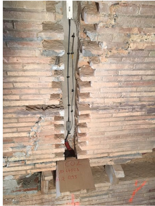
Figure 1. Optical Strand Strain sensor and temperature gauge integrated inside the cladding of the Pont de Pierre in Libourne, France. The picture is taken before completion of the cladding. ©OSMOS Group SA.
