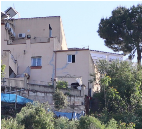
Figure 9. Cracks in a build from the northeast slope sector. The shown wall is oriented N145°E (northwest to the right). Other cracks can be seen in different walls of the same construction, not visible in the picture.
