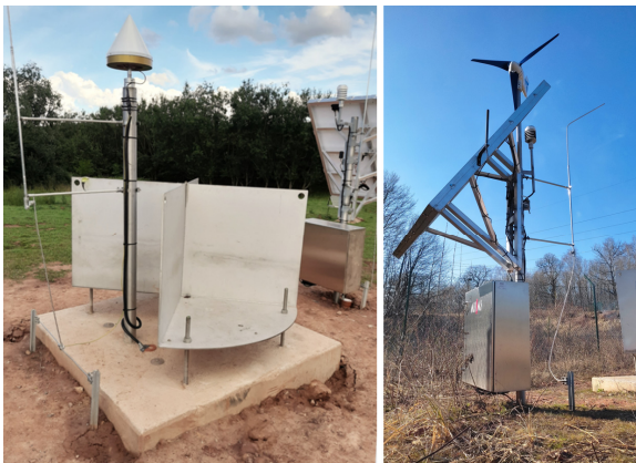
Figure 7. RAG's MSST Primsschacht (left) and solar & wind power supply on RAG's MSST Lauterbachschacht (right). Image courtesy ALLSAT & RAG.
