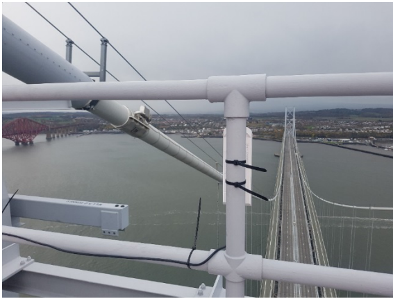
Figure 5. A TP-Link Wi-Fi transceiver point (CPE510) installed atop the NE tower of the Forth Road Bridge.
