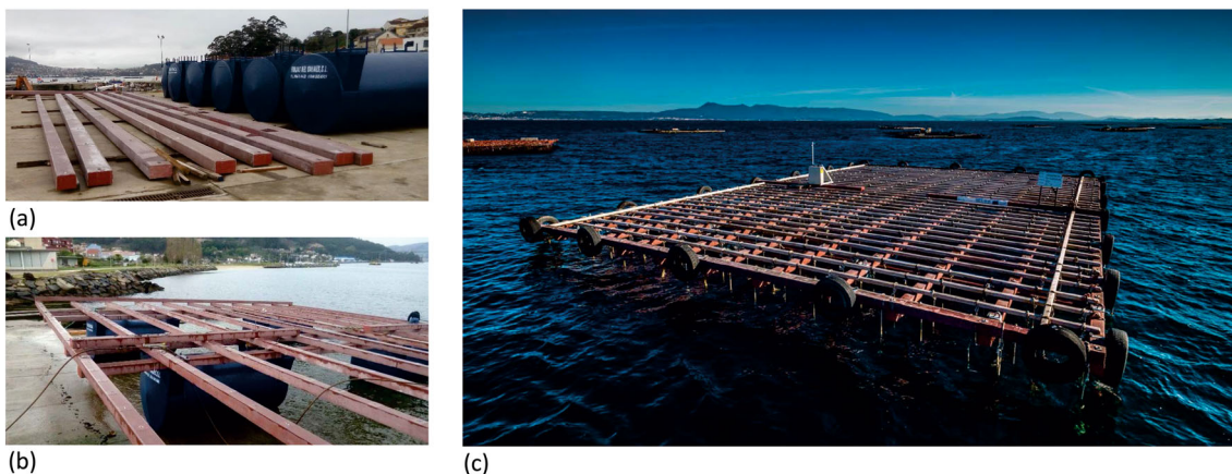
FIGURE 1 (a) UHPFRC beams (main and secondary) and floaters stored for assembling, (b) assembling process and (c) completely assembled offshore raft operating in the Arousa estuary (Pontevedra, Spain)
