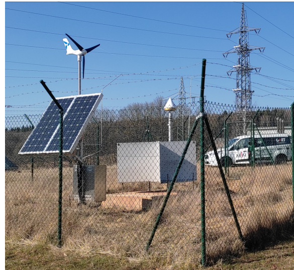
Figure 3. RAG's MSST Primsschacht for Saarland's SaarBoBeKa. From left to right: wind & solar power supply, equipment box, reinforced concrete foundation block at size 2 m x 2 m x 2 m, D-CR Ø2,0 m, JAVAD RingAnt-G3T GNSS chokering antenna. Image courtesy ALLSAT.
