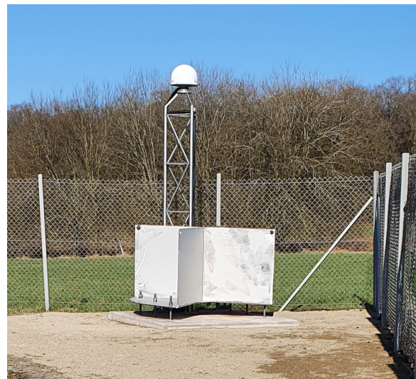
Figure 1. LVGL's MSST Hellendorf for Saarland's SaarBoBeKa on a deep and solid grounded reinforced concrete foundation 2 m x 2 m x 2 m, Leica AR25 GNSS chokering antenna, D-CR Ø2,0m and levelling points in foundation. Image courtesy LVGL.
