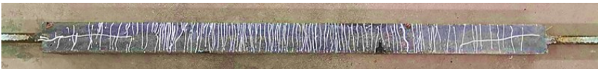
Figure 6- 31: A large number of the microcracks along the tensile R-UHPFRC element length.
