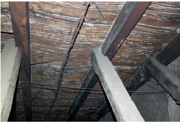
Fig. 15. Detail of the reed roof over trusses on the roof deck. (Source: The author).
