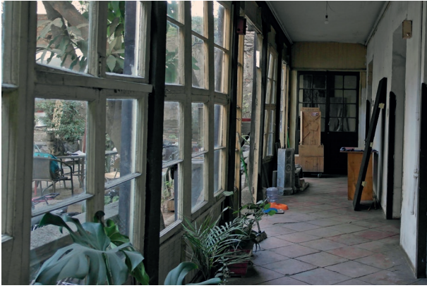
Fig. 20. Two-level volume corridor, with damage to the wooden pillar. (Source: The author).
