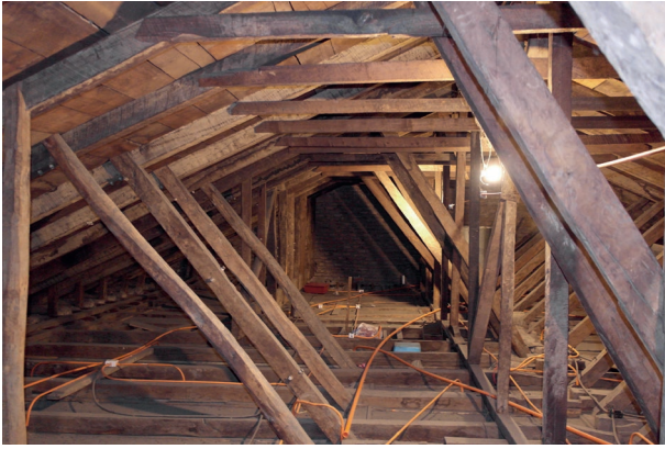
Fig. 14. Roof structure, wooden trusses connected to a chain in adobe walls. (Source: the author).
