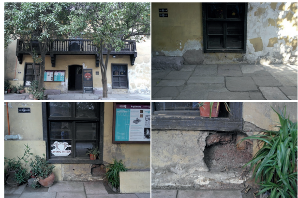
Fig. 19. Moisture damage to the base of adobe walls, main patio sector of the house. (Source: The author).
