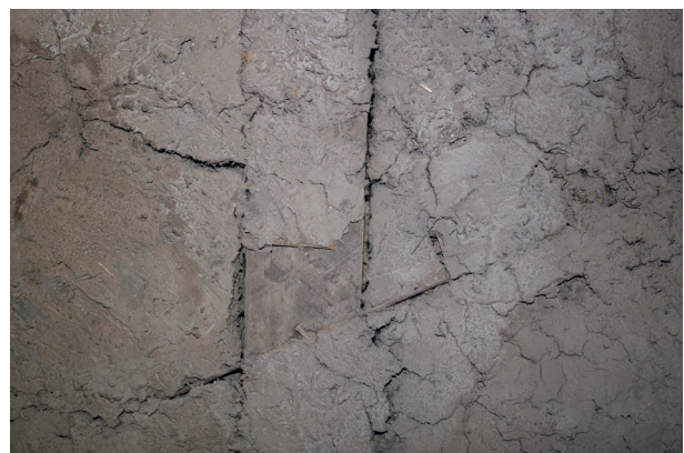
Fig. 13. Detail adobillo walls in the first floor and tower. (Source: The author).
