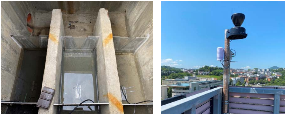
Figure 3: Three of the manholes built in Txomin-Enea. Weirs can be noted as well as the pressure sensors located in each manhole. Pluviometer installed on the roof of the School of Engineering of Gipuzkoa.
