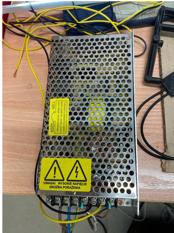
Figure 14. DC Motor Power Supply
