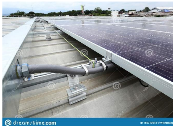
FIGURE 29 EXAMPLE OF THE METHOD INSTALLATION OF CONDUCTORS IN A CONDUIT OVER THE ROOF
