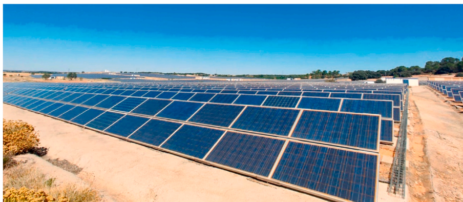
Fig. 2. Photograph of the PV plant.
