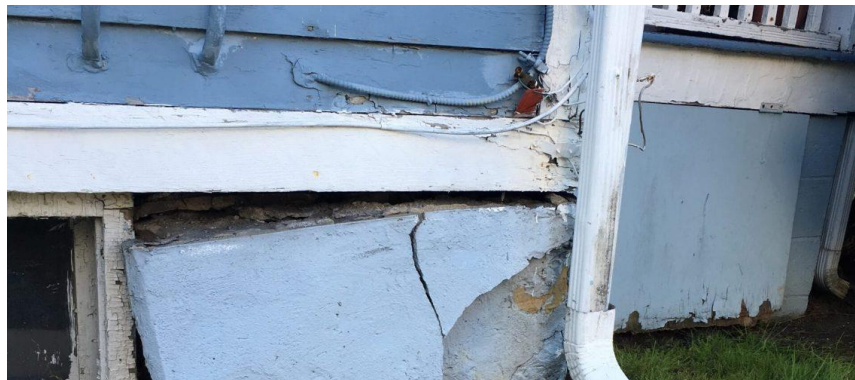
Figure 21. Withdrawal crack. Source: Effects of expansive soil on building (Lowy et al., 2022)
