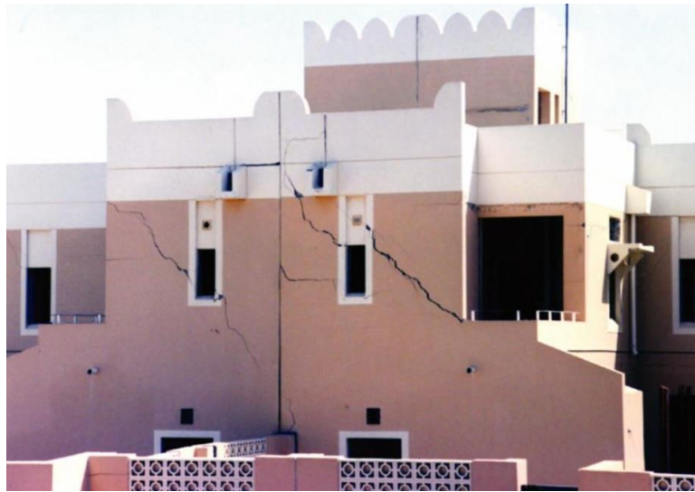
Figure 40. Severe case of cracking on the façade of a southern riad in Morocco. Source: Clay pathologies case studies (The constructor, 2009)
