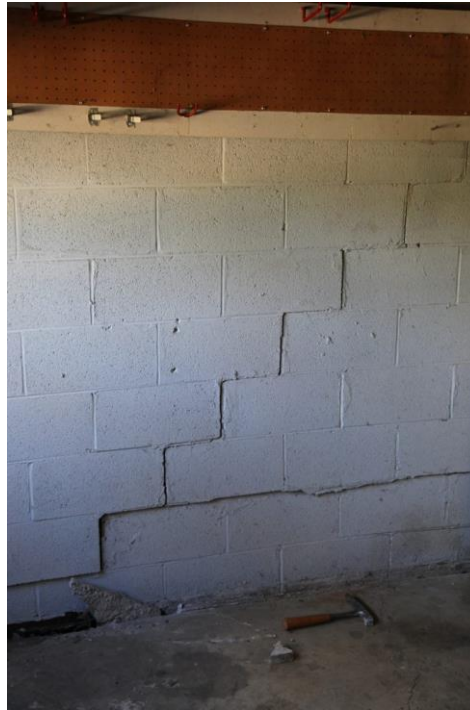
Figure 49. Damage on the stair bearing wall showing stair cracks. Source: Crack Patterns (United structural systems, 2023)
