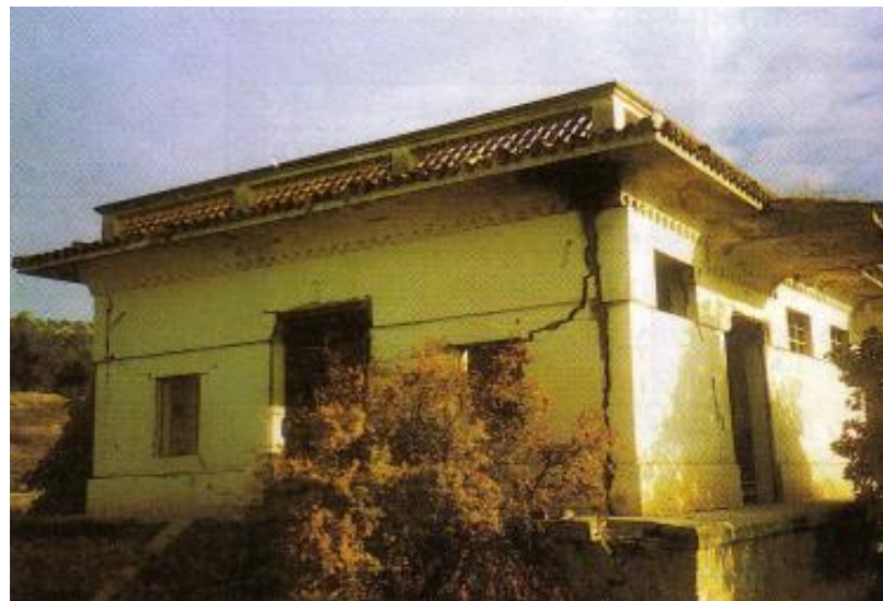
Figure 24. Example of a facade crack in Jaen. Source: Photo (Gonzalez Vallejo et al., 2002)
