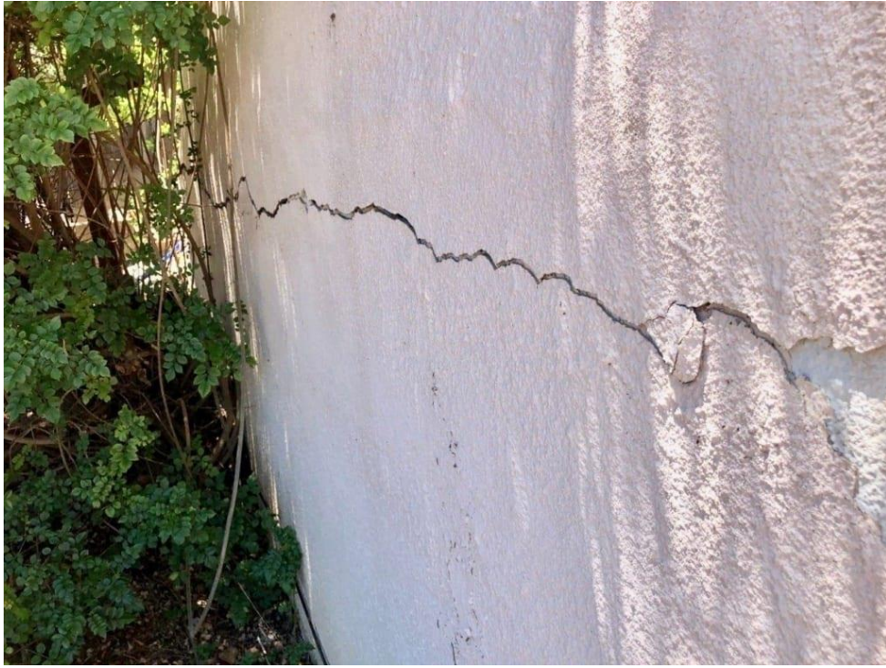
Figure 51. Facade crack. Source: Common Bay Area Foundation Problems and Their Solutions (Egloff, 2019)
