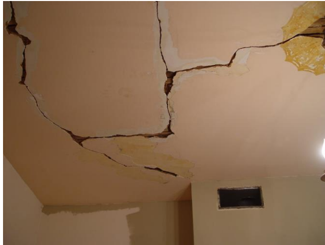
Figure 23. Example of a spider web crack. Source: Ceiling cracks and settlements (Gohl, 2022)
