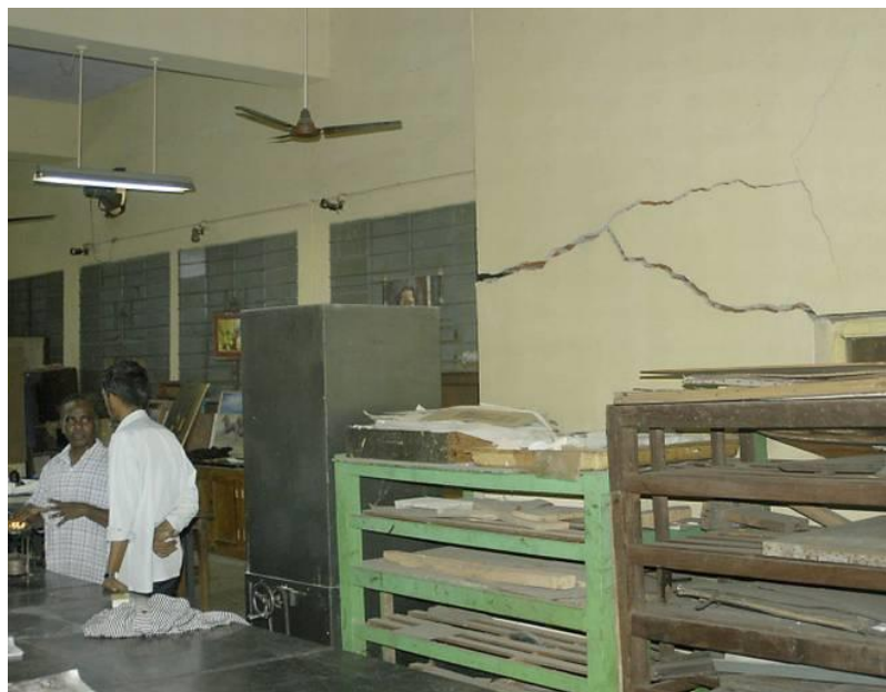
Figure 41. High risk observed crack on the basement wall. Source: Reasons why buildings crack (Prathima Seethur, 2018)
