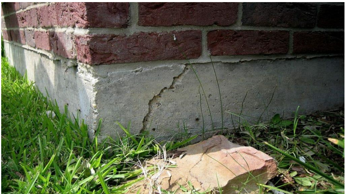
Figure 50. Crack due to bad settling because of clay swelling. Source: Foundation Problems vs. Settling (Flicker, 2022)
