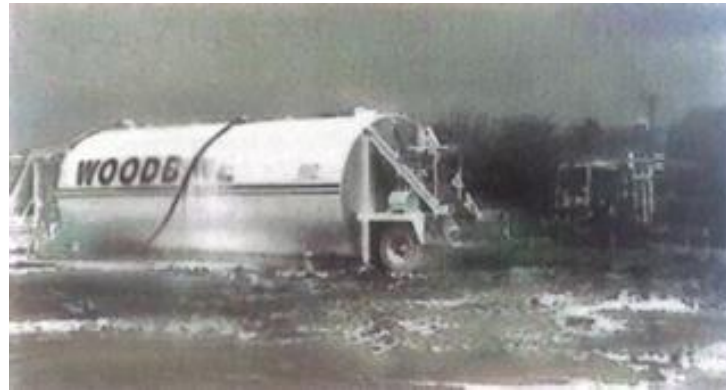
Figure 64. Pressure injection of lime slurry for a building pad (Hayward Baker). Source: Foundation engineering ( M.das, 1984)
