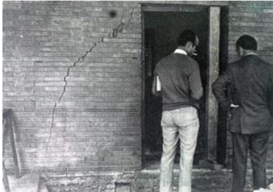
Figure 46. Settling produced due to the inundation of expansive clays (Breakage of pipes). Source: Geoténica y cimentos (Jimenez Salas, 1999)
