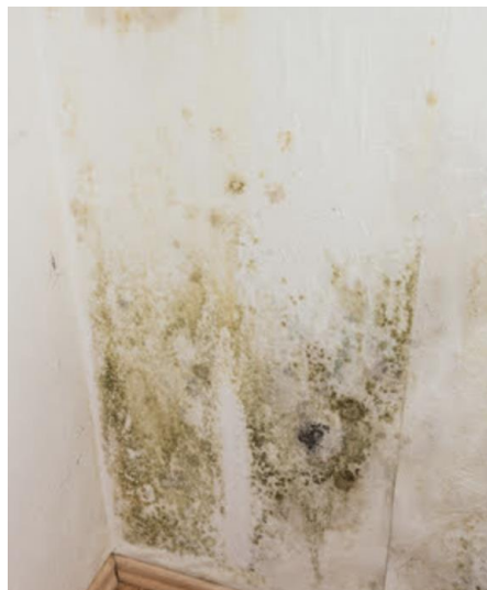
Figure 48. Mold growths on a corner of the wall due to water infiltration. Source: Reparations of humidity consequences (Valleywide, 2000)
