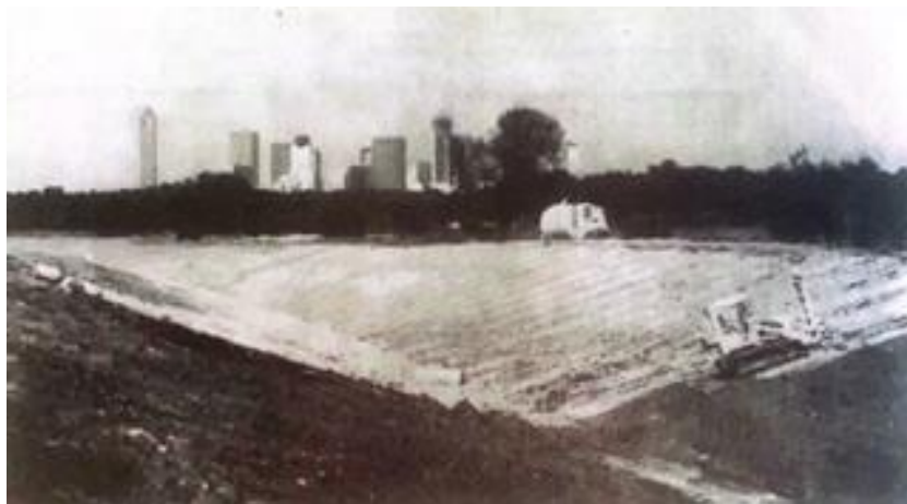
Figure 59. Slope stabilization of a canal bank by pressure injection of lime-ash slurry (Hayward Baker, inc). Source: Foundation engineering (M.das, 1984)
