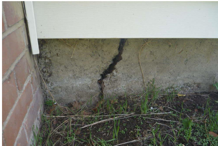
Figure 42. Upheaving of the basis of a house. Source: A case scenario of a failure of foundation (Parathima Seethur, 2018)
