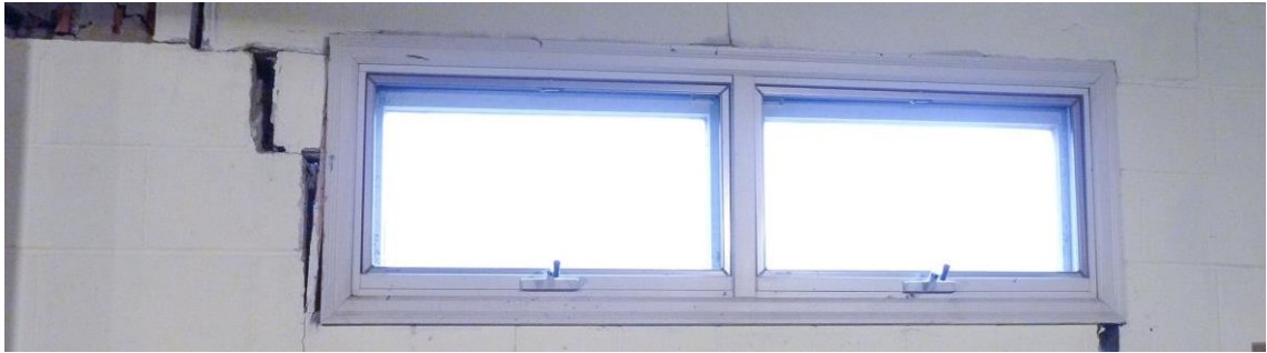
Figure 44. Apparition of severe cracks and frame distortions. Source: Foundation Wall Repair in Northwestern PA (Total foundation inc, 2014)
