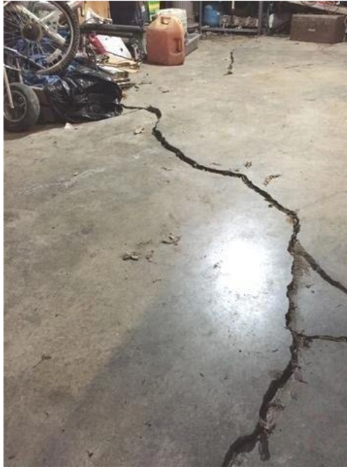
Figure 47. Damage on the pavement of a garage due to expansive soils. Source: Expansive soils (Property health inspection, 1999)
