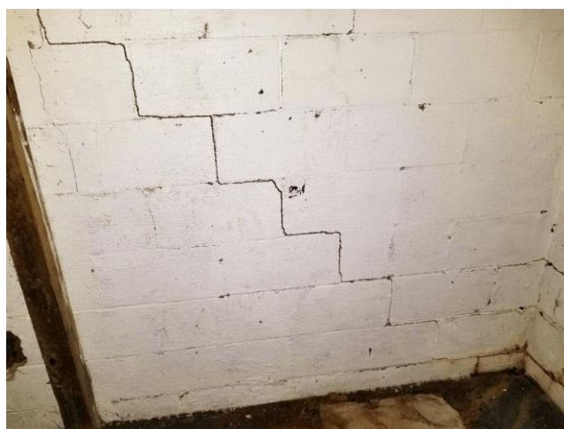
Figure 22. Example of stair crack in Georgia. Source: Foundation cracks and the damage they cause (Contreras et al., 2022)
