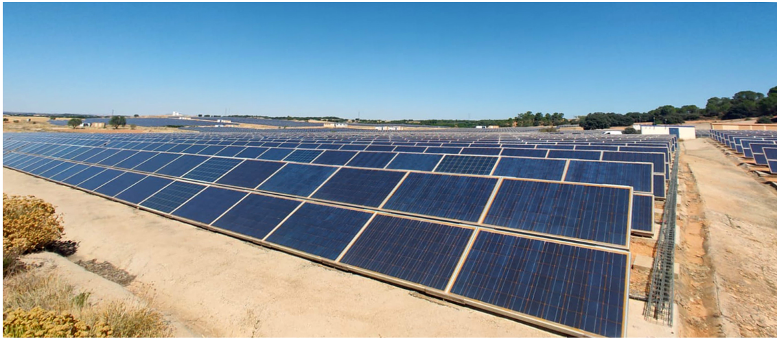
Figure 2.2: Photograph of the PV plant.
