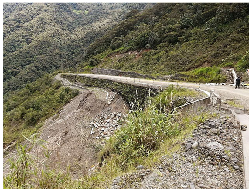
Figure 2. A view of the middle part of the landslide area where the road was affected (cut) and reconstructed, applying observed earth-walls. In this location, the movement is prone to continue at a low displacement tax. The high slope on the landscape can be observed.
