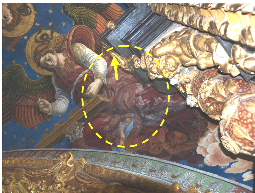
Figure 7. Picture of the fresco painting where sensor AB is located (exact position indicated with an arrow). The dashed ellipse highlights a zone with white salt efflorescence stain. The picture was taken in March 2011.
