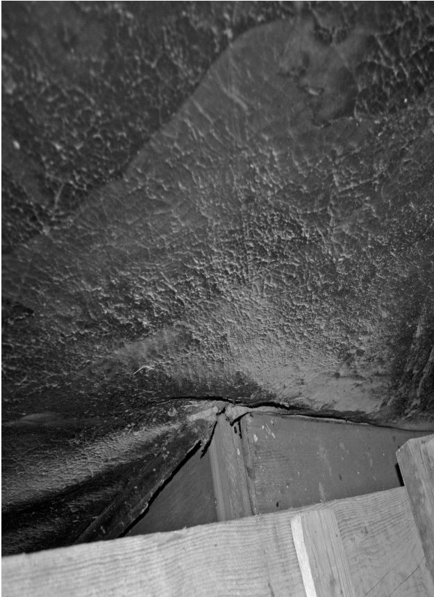
Figure 5. Deposits of dust detail and paint distortions
