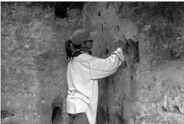
Figure 10. Cleaning and consolidation of stucco on the palace walls of La Blanca
