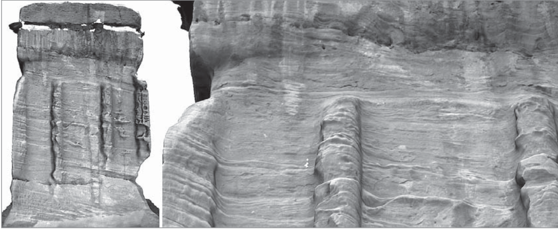
Figure 9. General view and detail of a photorealistic 3D model of the southern elevation, 2010. (GIFLE)
