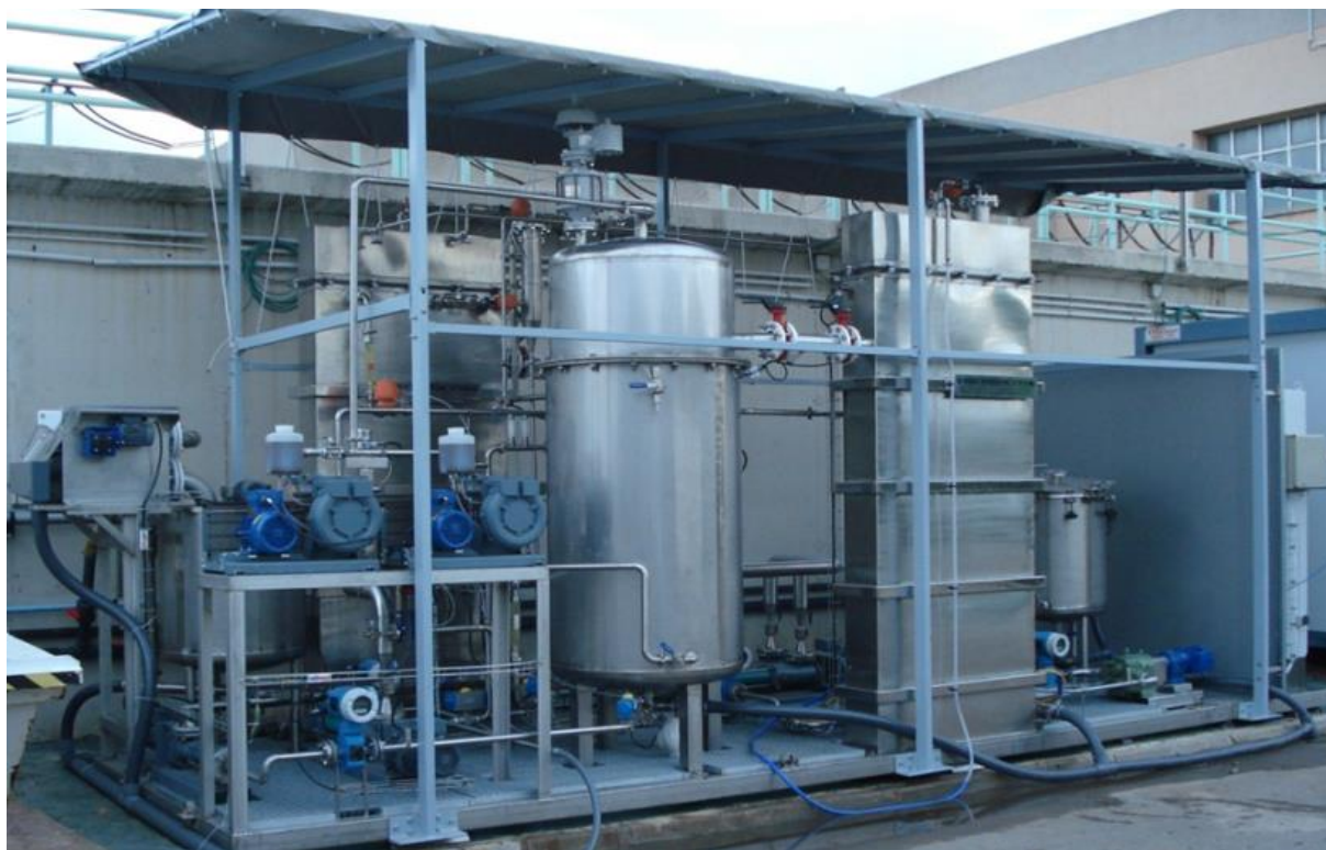
Figure 3.1 General view of the SAnMBR demonstration plant.
