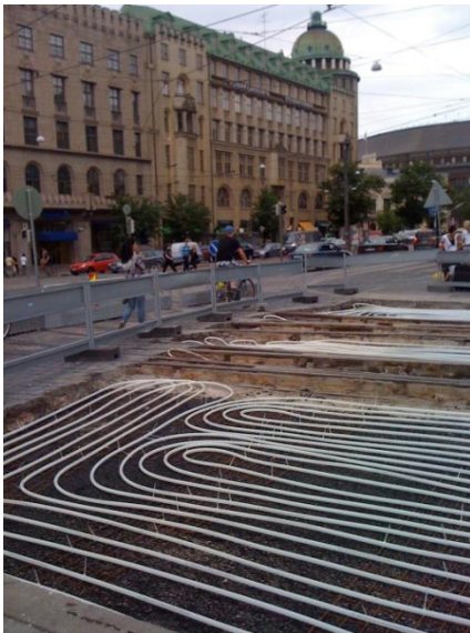
Helsinki Street with under floor heating [1]
