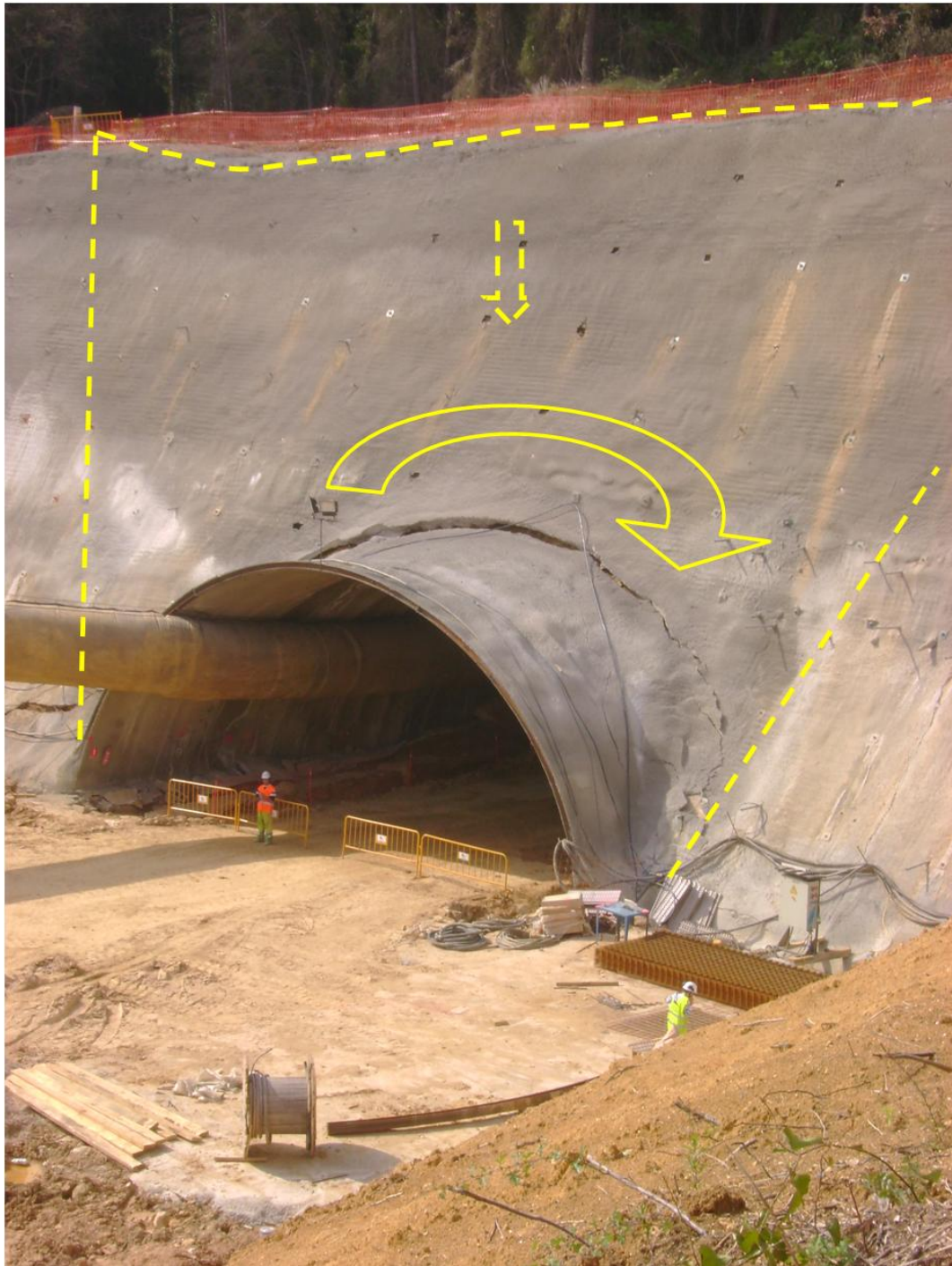
Fig. 6 Overview of the North portal after the collapse. The horizontal dashed line highlights the 0.5 m depression at the top of the portal. The dashed harrow points the downward movement. The vertical and inclined dashed lines indicate the two longitudinal fissures 30 m long, The circular arrow indicates the circular shape of the fissure above de tunnel lining
