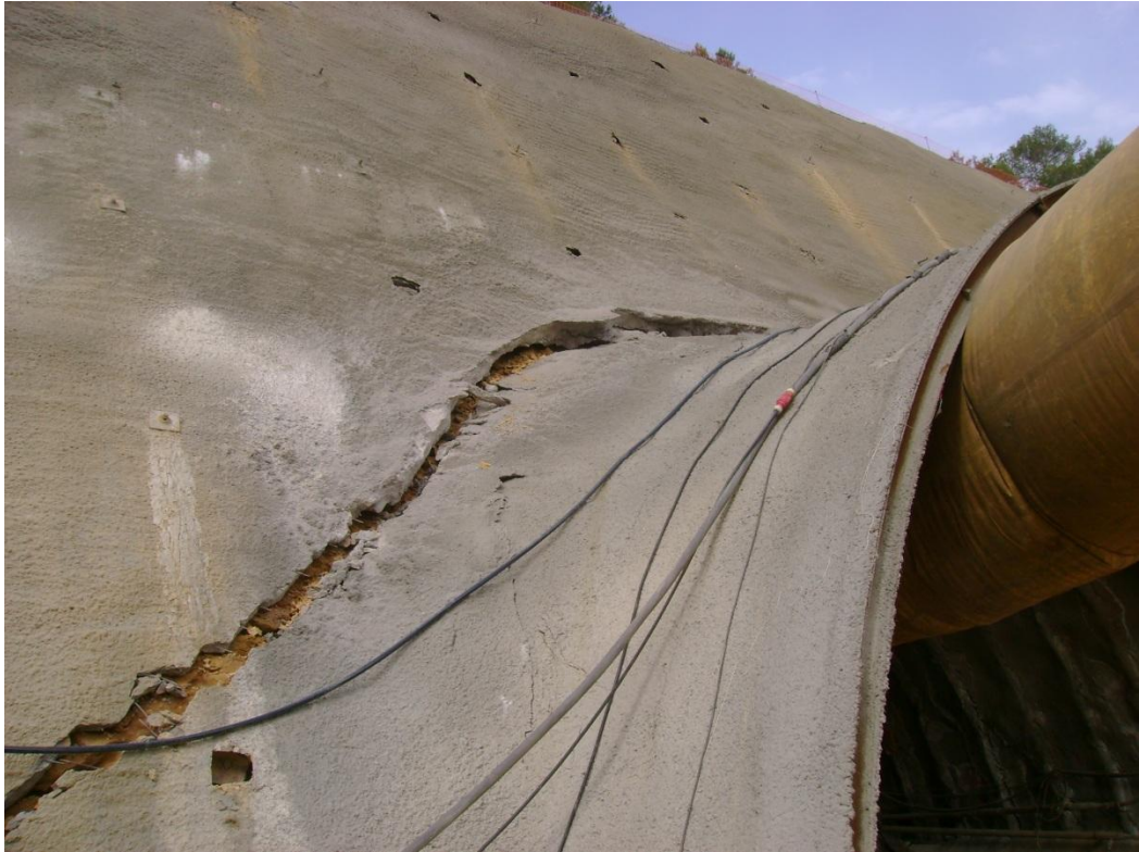
Fig. 7. Fissure developed above the North portal lining.
