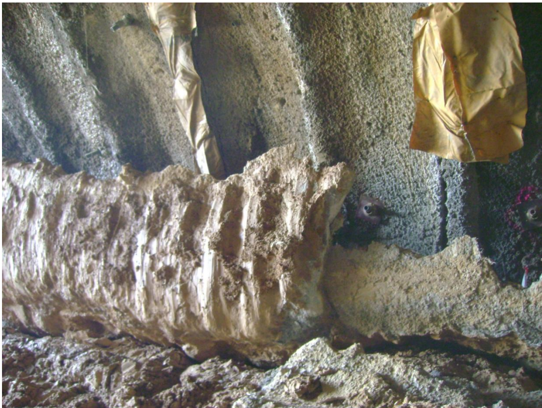
Fig. 8 View of the provisional mortar gutter rotated upwards on the left side of the tunnel
