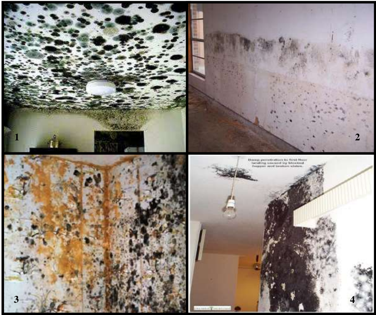
Fig.3.3. Representative pictures for “Damp and Mould” hazard
