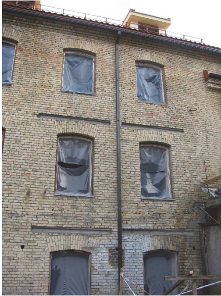
Figure 67. Facades of courtyard before the reconstruction works. 1st phase replacement of the lintels is done.
