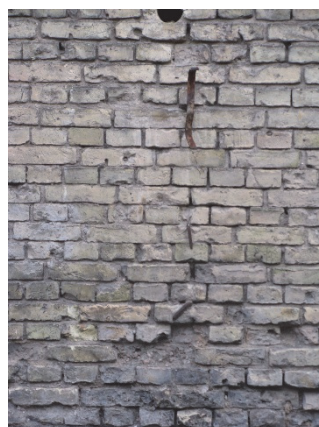
Figure 39 . Example of crack and rests of rusty iron in courtyard wall
