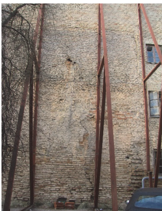
Figure 40 . Example of crack in wall
