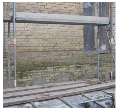
Figure 38 . Example of moisture in courtyard wall
