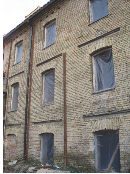
Figure 68. Facades of courtyard before the reconstruction works. 1st phase replacement of the lintels is done.
