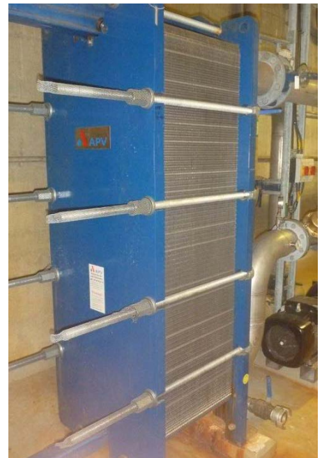
Figure 5.5: Picture from Oset WTP (Plate heat exchanger,
