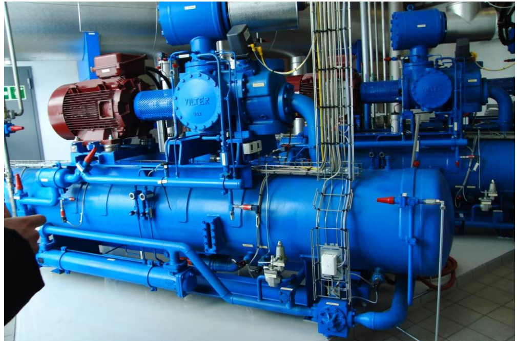
Figure 5.2: Picture from Hias WWTP (the heat pump compressors)
