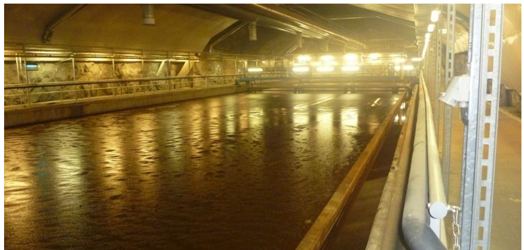
Figure 5.8: Picture from Bekkelaget WWTP (Activated Sludge system)
