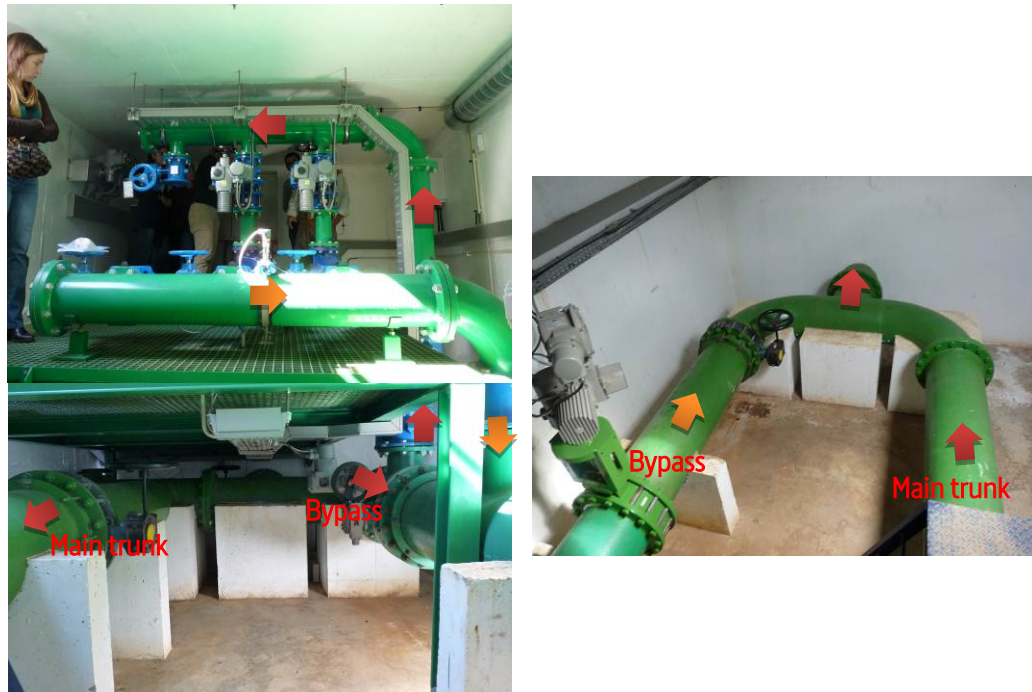
Figure 10.2: View of the bypass inside the valve chamber
