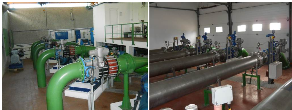
Figure 3.1 Reversible pumping station
