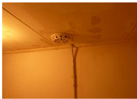
Image 12.2-5 Fan of the washing machine room from the first floor (room 14)
