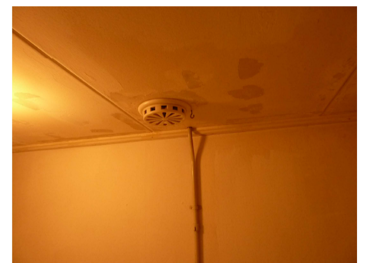
ROOM Nº14 MECHANICAL VENTILATION IN THE WASHING MACHINE AND DRYER ROOM
