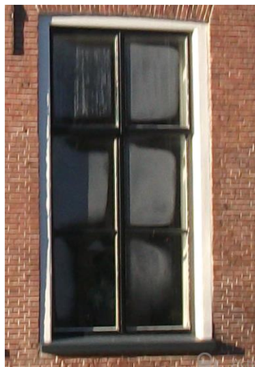
Image.9.1.1-1- Surface condensations on one window from the main facade of the ground floor.
