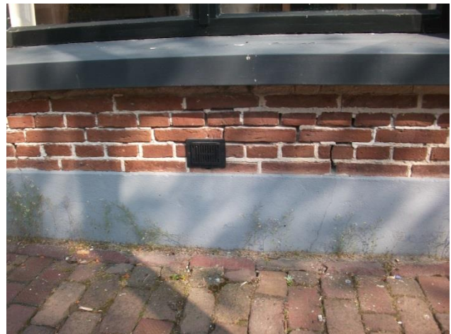
Image 10.2.6-4 Cracks window C
