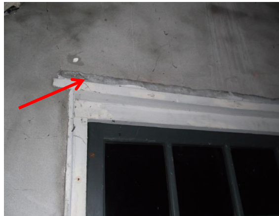
9.1.2-2 Different solutions applied to the air leaks: paperboard and insulation (attic of the building)
