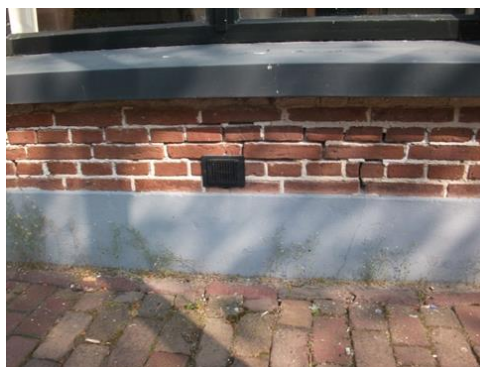
Imagen 9.2.3-1Crakcs of the main facade
