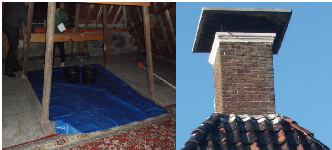
Image 9.2.2.-2 Water filtrations behind the chimney
