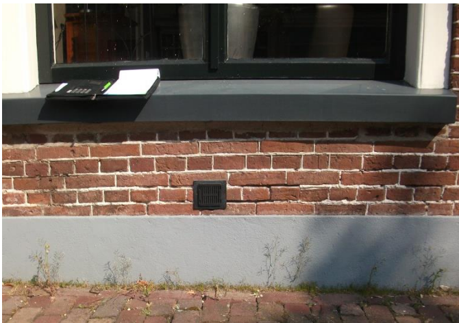
Image 10.2.6-3 Cracks window B
