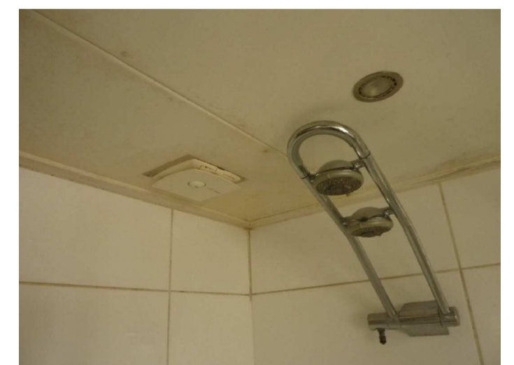
ROOM Nº17 MECHANICAL VENTILATION IN THE BATHROOM
