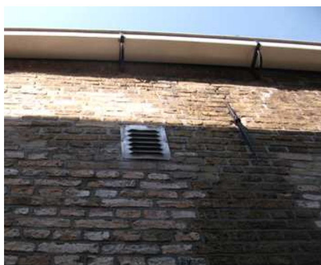
ROOM Nº9 METAL GRILL FROM KITCHEN HOOD VENTILATION
