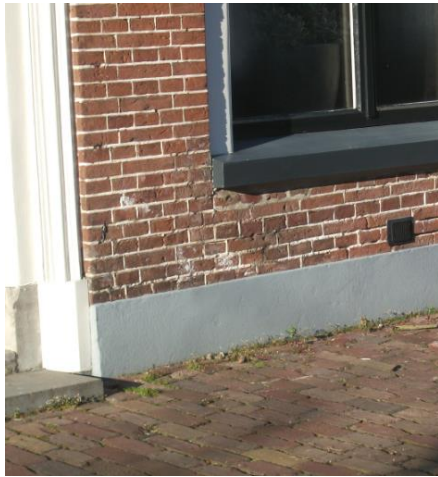
Image 9.2.2.-3 Efflorescence on the main facade
