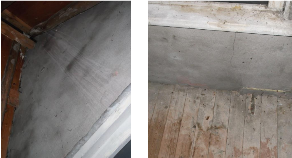
Image 9.2.2.-1 Moisture leaks at the attic
