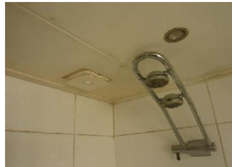
Image 12.2-4 Fan of the bathroom first floor (room 17)
