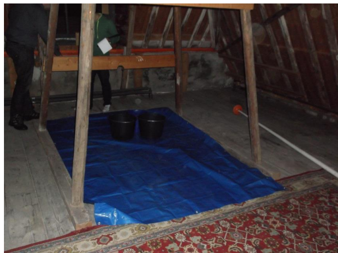
Image 4.4.-5 Water filtrations on the attic
