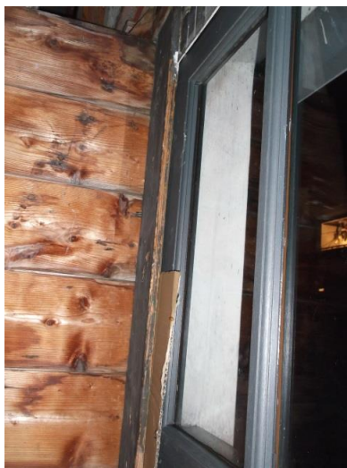
Image 4.4.-4- Air leaks attic window
