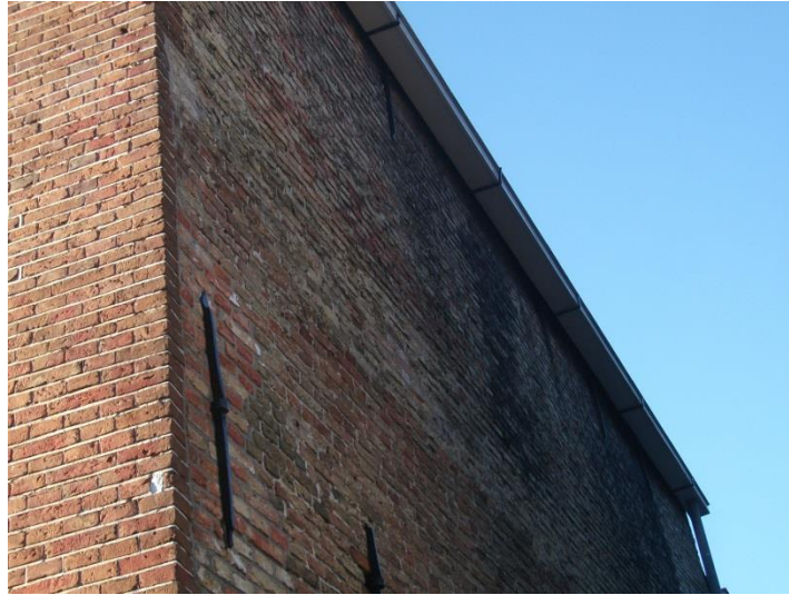
Image 9.2.2.-5 Moisture spots at the east facade
