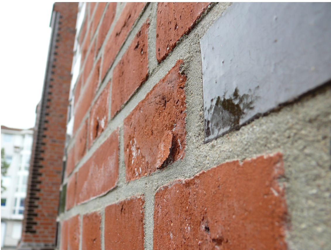
Pic. 3.2.1.4. Spalling brick.
