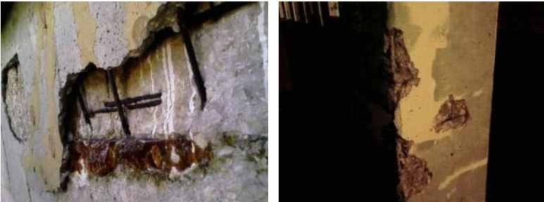
Structure of a storage tank with armour in sight (before repair)
