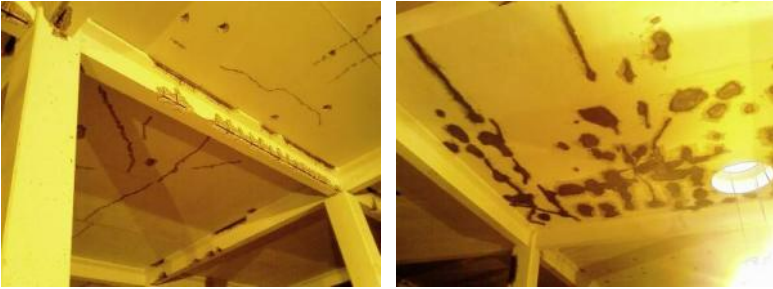
Coverage cracks: before and after repair with cement mortar
