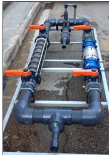
Figure 1. Pilot installed in the water network.
