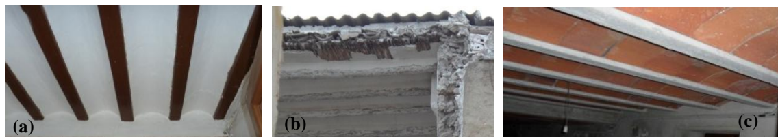
Fig. 7 Horizontal structures: a ) timber floors (timber beams and joists with lightweight masonry vaults), b ) roofs (reed and plaster deck, “cañizo”, under ceramic curved tiles) and c ) new RC floors (RC beams and joists with ceramic vaults)
