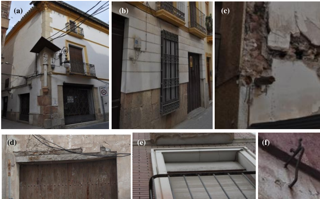
Fig. 9 Reinforcement elements: a) Quoins, b) Plinths, c) Floor and wall timber ties or timber ring beams, d) Timber lintels, e) Stone frames around openings and f) Iron ties
