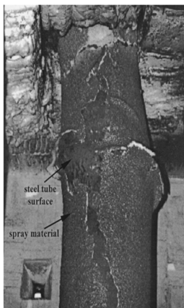
Figure 4.9. Typical failure of spray protection after fire tests (Han et al. 2003a).
