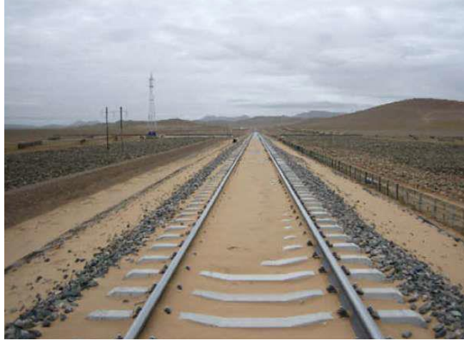
Figure 10. Example of track infrastructure covered by sand in China, [9]
